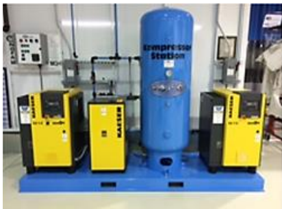
Pictured above: Duplex 7 1/2 HP w/ 120 gallon tank & Dryer
